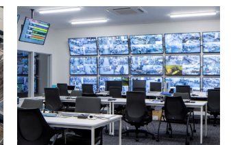
Control room of the Factory No. 3
